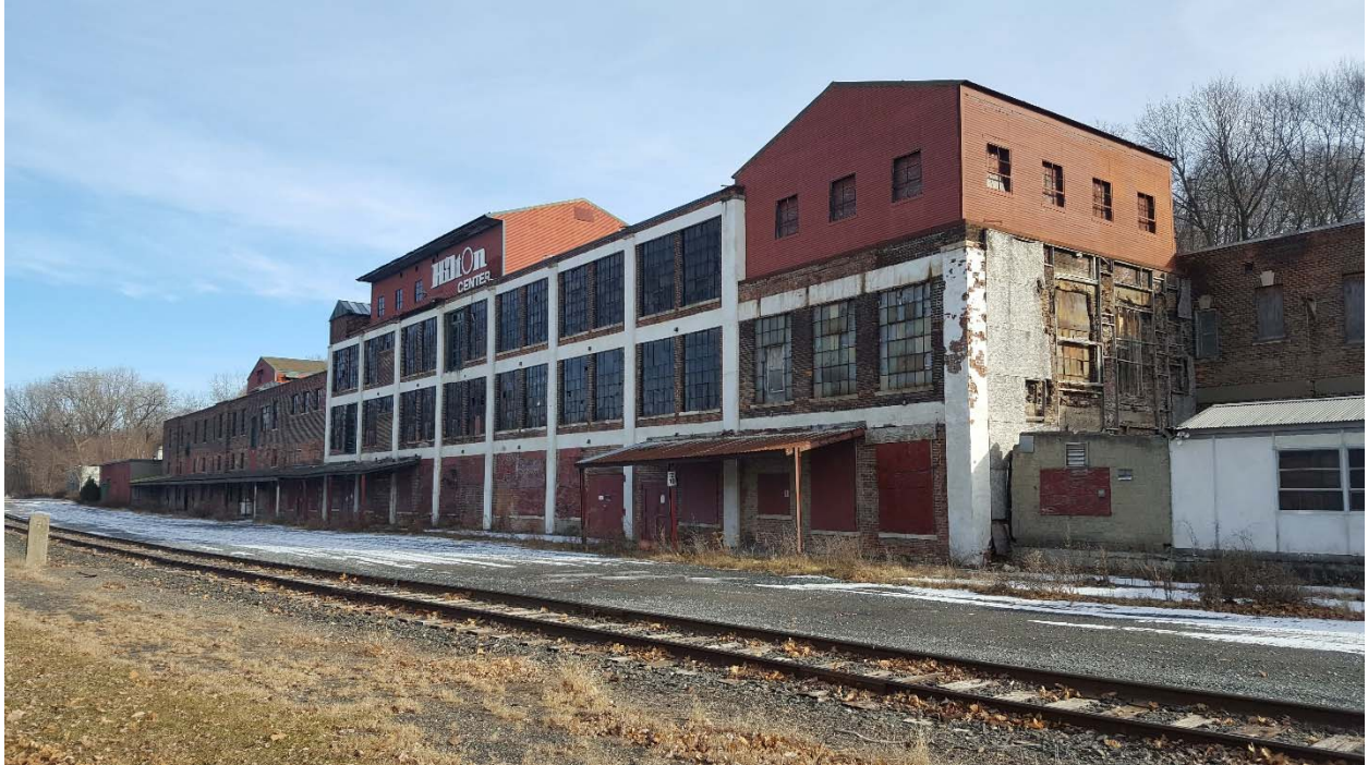
Photo 15. View northeast of the former William Barnet & Son's Shoddy Mill Complex (08341.001134), now known as Hilton Center.
