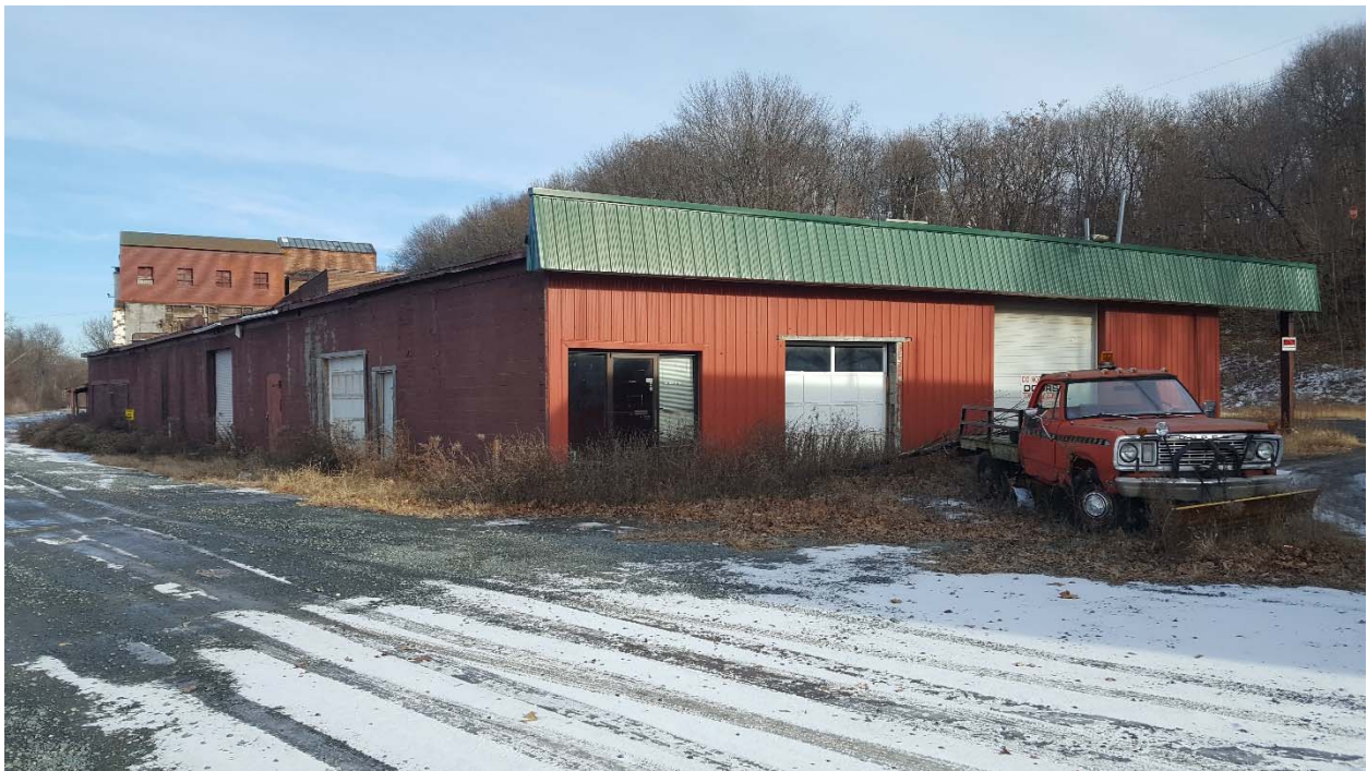
Photo 14. View east of a concrete or cinder block structure dating to between 1909 and 1949. The building was formerly used for rag storage. Part of the former William Barnet & Son's Shoddy Mill Complex (08341.001134).
